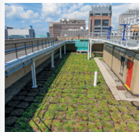
SUSTAINABILITY GREEN ROOFS INITIATIVE Green roof at 1133 Avenue of the Americas, completed in 2013.
