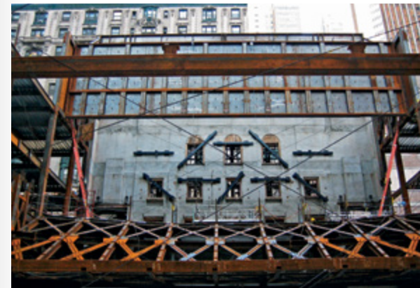
HENRY MILLER'S THEATRE RESTORATION Structural supports are used to keep the historic facade of the 43rd Street theatre intact while the interior is reconstructed during the 2005 restoration. The theatre officially reopened in 2009 with Roundabout Theatre's production of Bye Bye Birdie .
